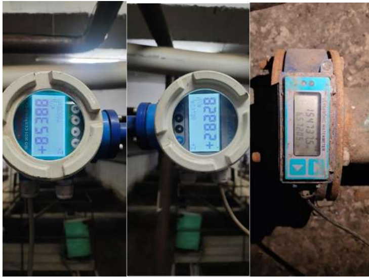
STP INLET AND OUTLET METERS
