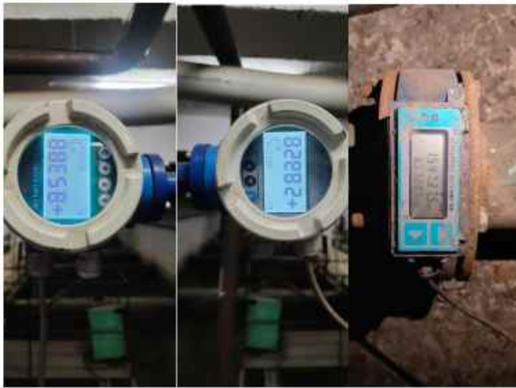
STP INLET AND OUTLET METERS
